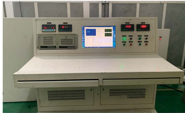
Fan performance test data acquisition system
